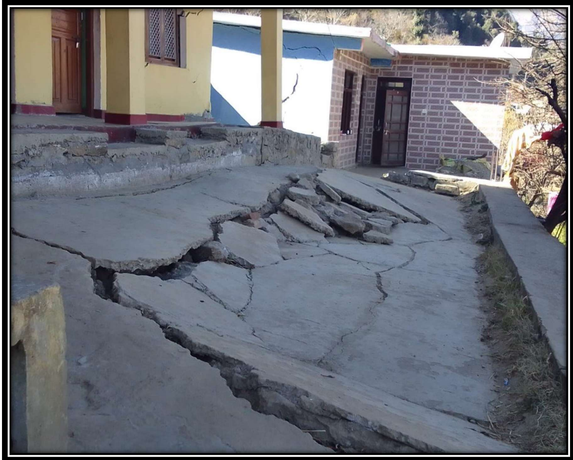
Image 1.4: Showing Cracks in the houses of Joshimath
