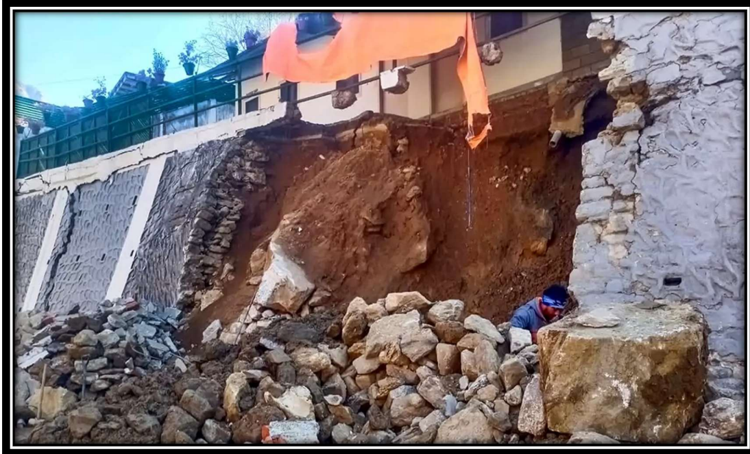
Image 1.3: Landslide at Joshimath
